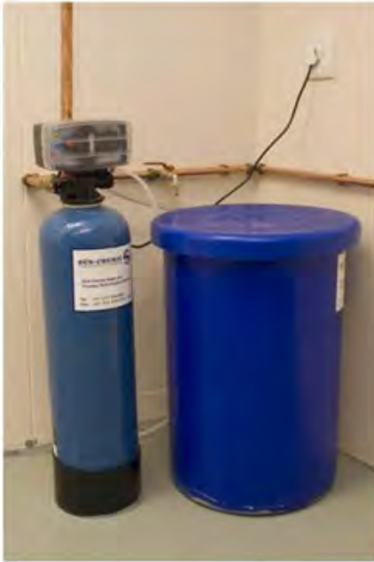
SPT 20 UNIT – Water softening system
