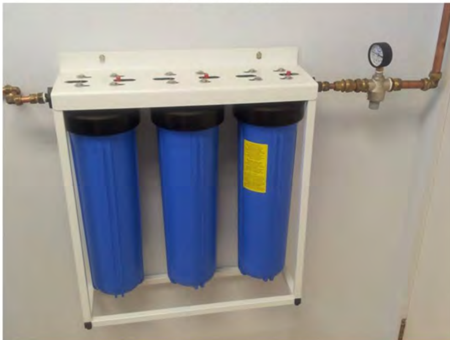
Big Blue water filter system
